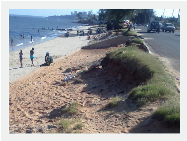
Image 18: Av. Marginal before (left) and after (right) CMM intervention. Source: Google Images.
